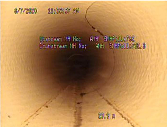
Figure 10 - Spiral Fracture in Overflow Pipe
