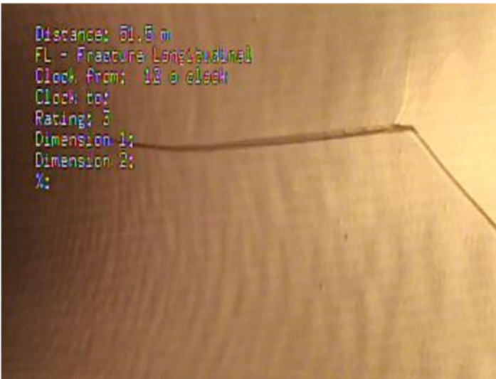
Figure 9 - Longitudinal Fracture in Overflow Pipe
