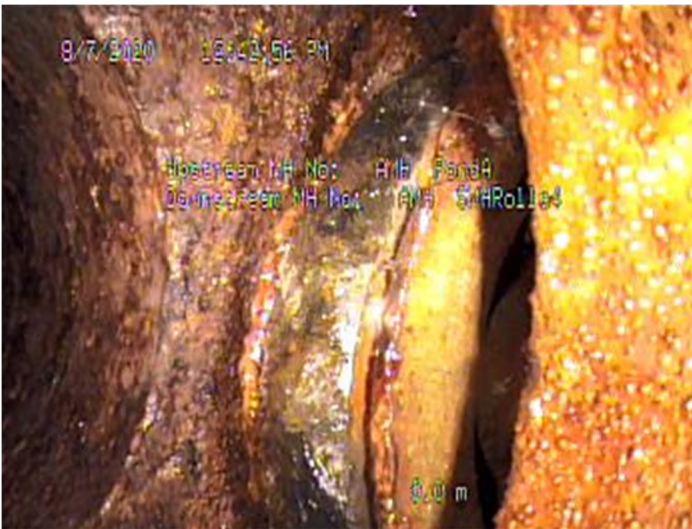
Figure 12 - Severe Corrosion in Valve Between Lagoons
