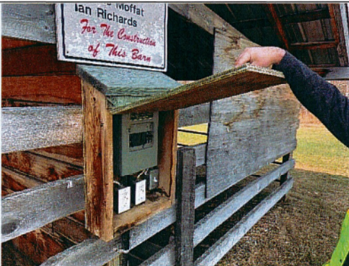
Unlocked not weatherproof panel enclosure
