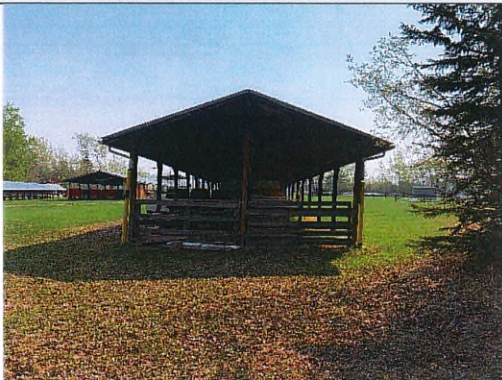
Leaning (long pole barn)
