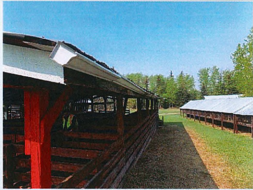
Gutters in poor condition
