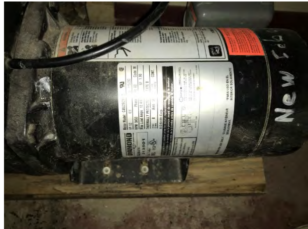
Domestic water booster pump
