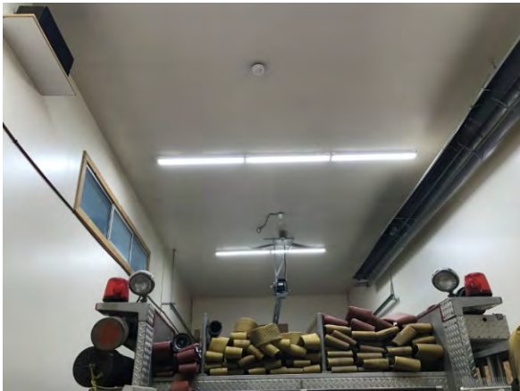
Fluorescent T8 Lighting in the facility
