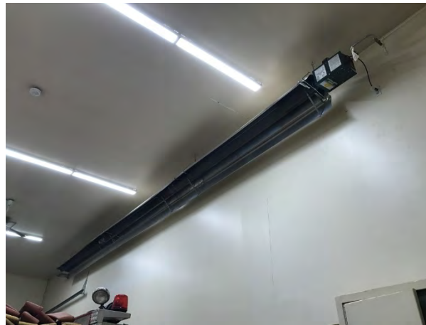
Propane fired radiant tube heater
