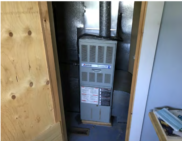
Main heating boiler
