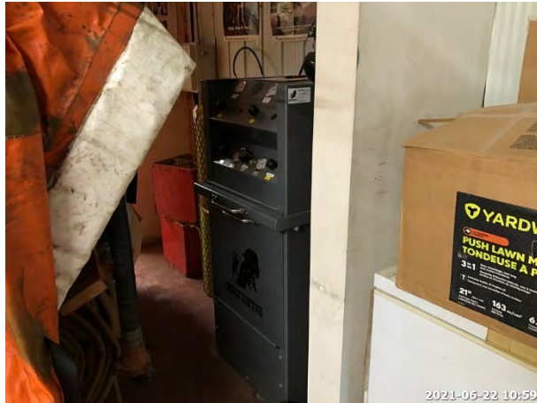
Breathing air generator
