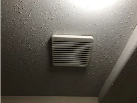
View of ceiling mounted bathroom exhaust fan
