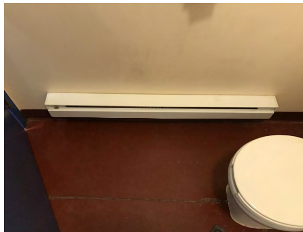
Typical electric baseboard heater in the washrooms
