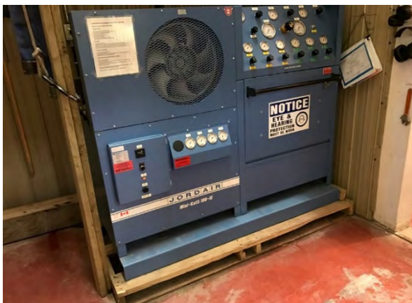
Breathing air generator
