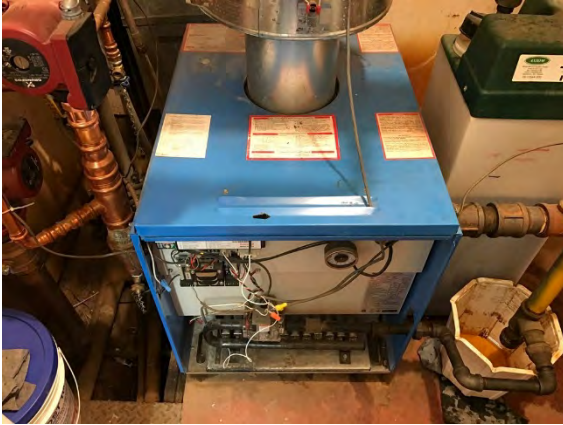
Main heating boiler
