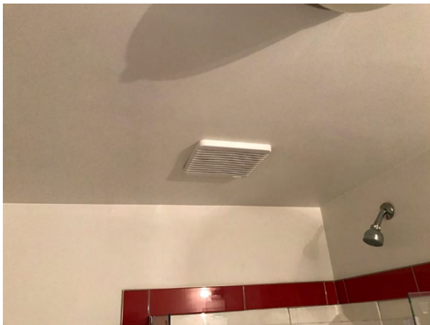
View of ceiling mounted bathroom exhaust fan
