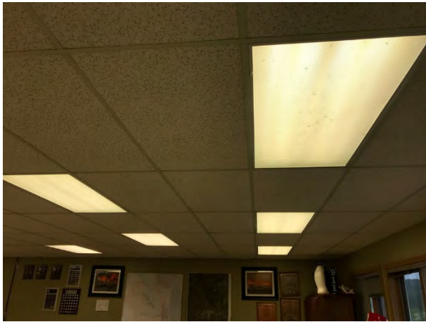
Fluorescent T8 Lighting in the facility
