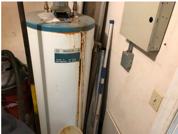
Natural gas fired DHW heater
