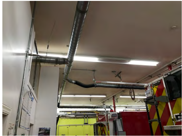
Newer LED lighting in the Apparatus Room
