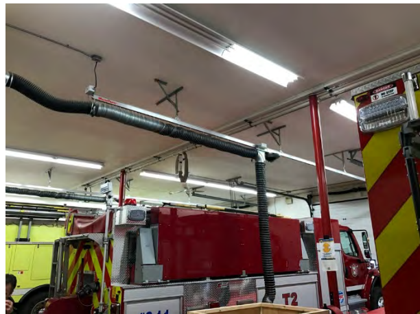
View of the apparatus hall exhaust air system
