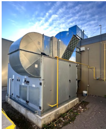
Figure 11: Munters Dehumidification Unit
