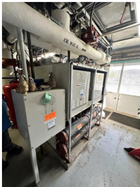
Figure 12: Existing Multistack Unit
