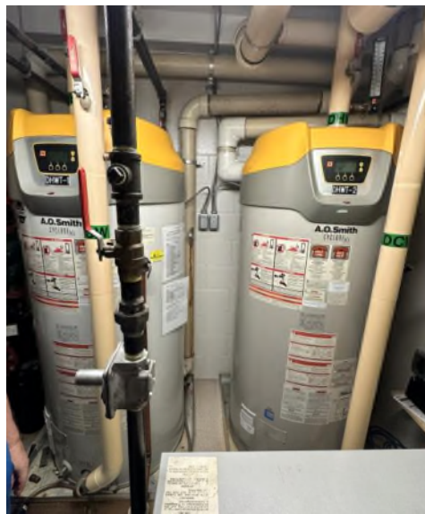
Figure 8: A.O. Smith Water Heaters for Arena-DHW Heating
